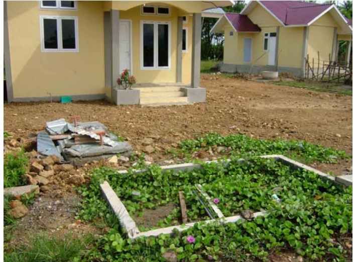
Faults: Unnecessary vents Outlet lower than inlet Soil in wetland
