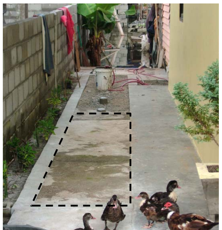
Above: Half of this ARC/BRCS wetland & vegetated leachfield system has been concreted over rendering it non-functional.
