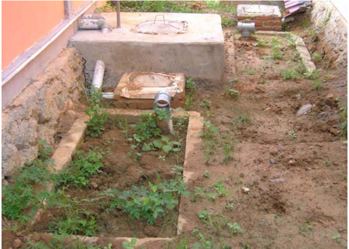
Above: Poorly constructed wetland system ARC ARC/BRCS Wetland system, no plants
