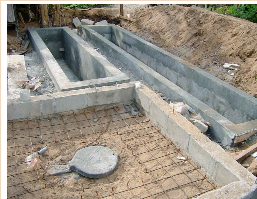
Fiberglass septic tank 1,000l under concrete slab 2m x 2m
